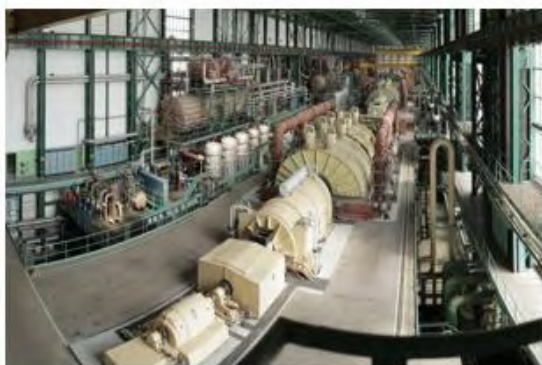
Turbine hall before any dismantling (05/2013)
