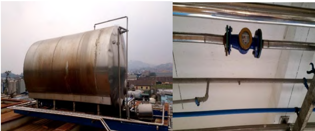
A recovery tank installed to recover cooling water and a meter installed to measure recovered water
